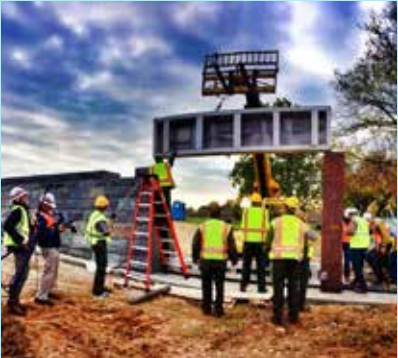
17th Street, NW Levee Installation Photo Credit: U.S. Army Corps of Engineers Baltimore District
