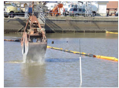
A crane placing materials as a part of a sediment capping experiment.
